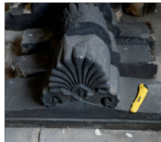
Some of the Alexander 'Greek' Thomson-designed details are crumbling
